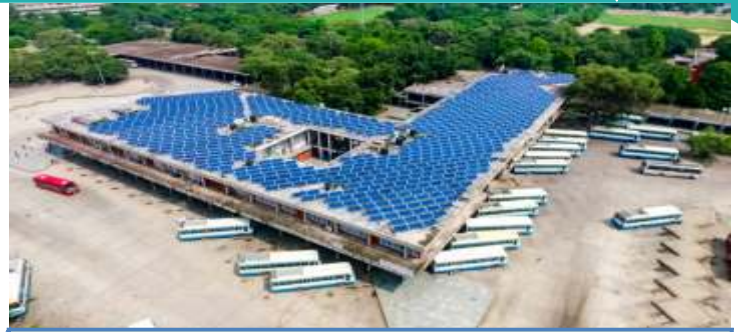
300 kWp Rooftop Solar Plant at ISBT, Sec17
