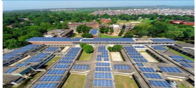
1000 kWp Rooftop SPV Plant at PEC, Sec 12
